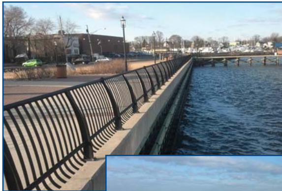
Wall After Hurricane Sandy
