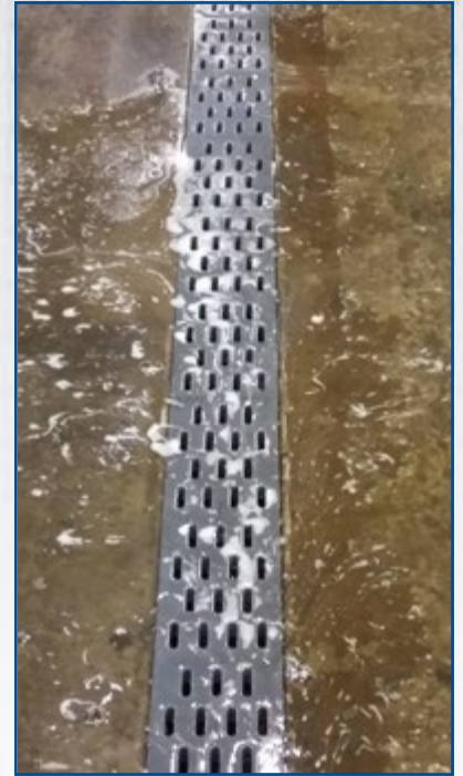
Finished In Use Corrosive Environment
