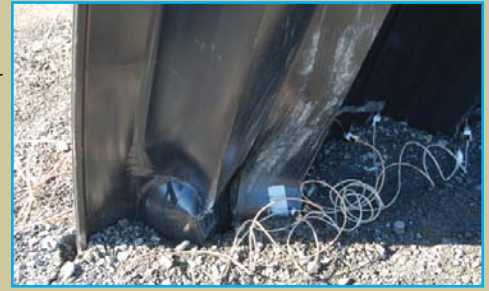
Example of Local Compression Buckling
